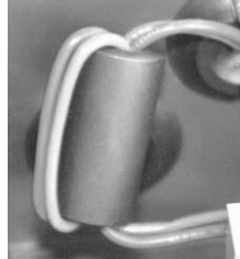
Figure 2-5: Ferrite core and battery supply wiring
